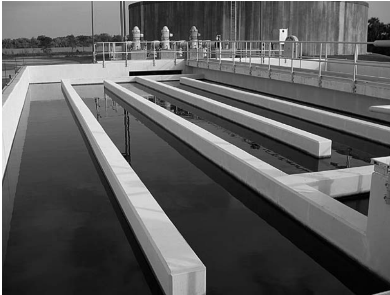
Figure 16.53 Serpentine chlorination reactor for wastewater effluent disinfection.
