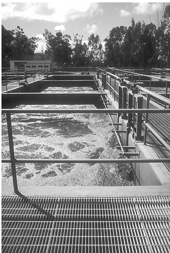
Figure 16.18 Suspended-growth (i.e., activated sludge) wastewater treatment facility.
