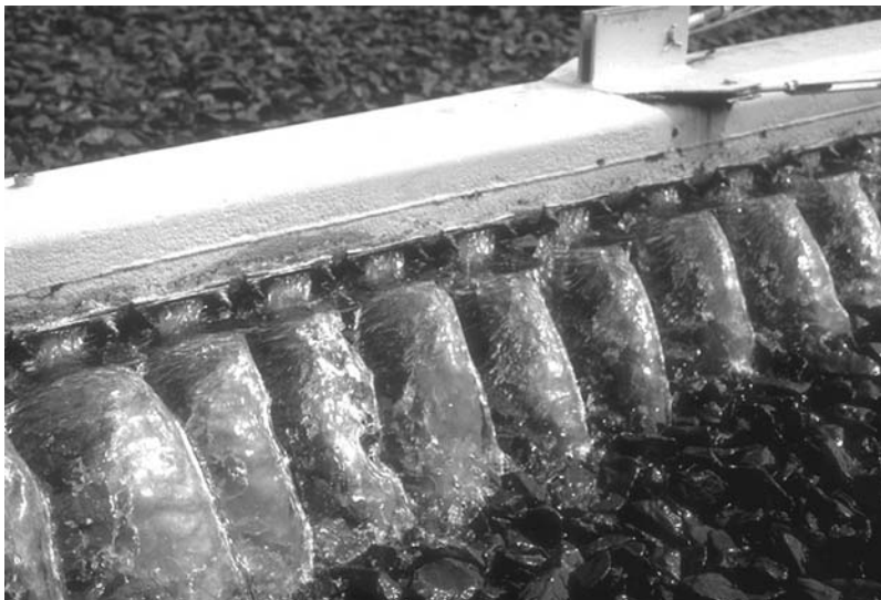
Figure 16.7 Attached growth wastewater treatment distributor.
