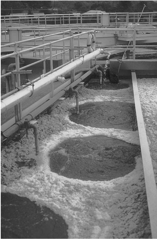
Figure 16.47 Aerobic sludge digestion system.
